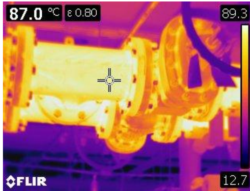
Figure 3 This thermographic image is of bare heating supply lines and valves at 87° C or 188° F.
