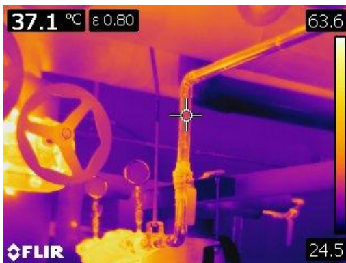
Figure 23 Thermographic image of a copper line from heating pump at 37.1° C or 98° F.
