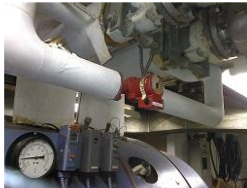
Figure 6 This conventional photo shows the same re-circ pump at the boilers.
