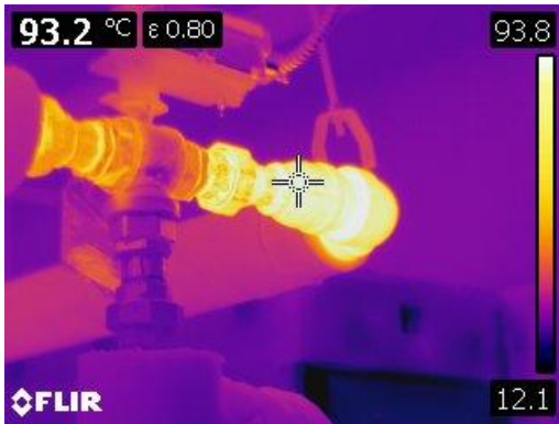
Figure 29 Thermographic image of bare motorized Tee at 93.2° C or 199° F.
