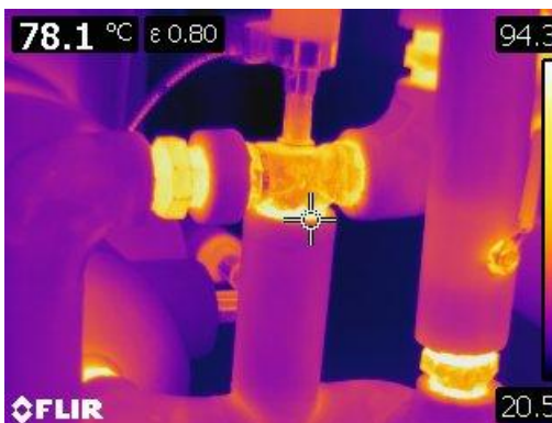
Figure 11 Thermographic image of bare motorized tee and associated fittings at the hot water tanks at 78.1° C or 172° F.
