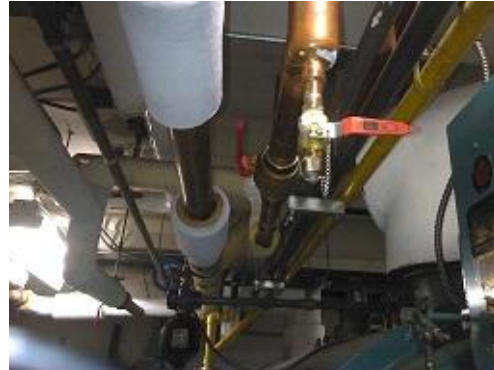
Figure 26 Conventional image of the same copper piping and valve.
