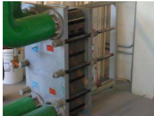
Figure 2 This photo shows the same plate heat exchanger.
