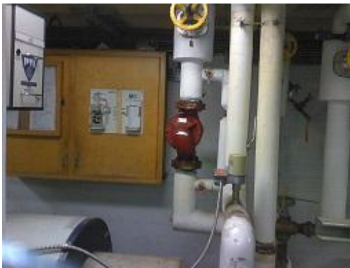
Figure 16 Conventional image of the heating pump.
