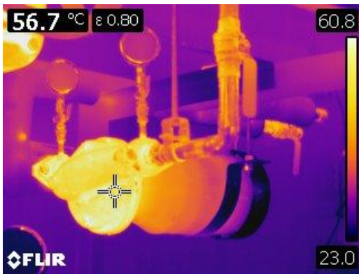
Figure 21 Thermographic image of a motorized heating pump at 56.7° C or 134° F.
