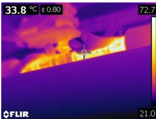
Figure 33 Thermographic image of motorized valve and pipe at 33.8° C or 92° F .
