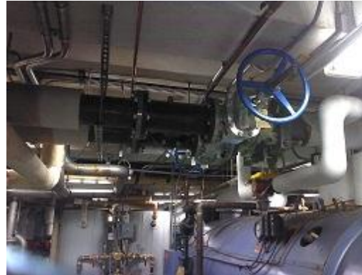
Figure 4 This is a conventional photo of the same piping and valves from the boilers.
