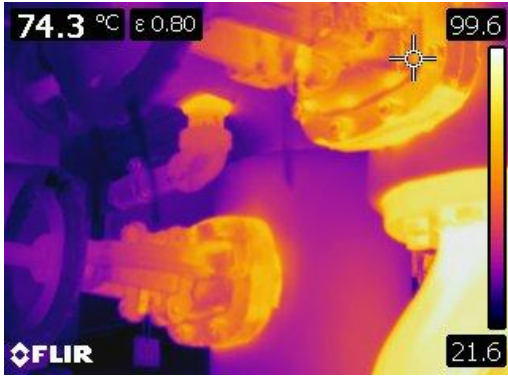
Figure 13 Thermographic image of bare valve bonnets on the heating supply at 74.3° C or 165 F.
