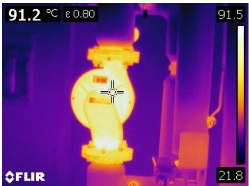
Figure 15 Thermographic image of a motorized heating pump at 91.2° C or 196 F.
