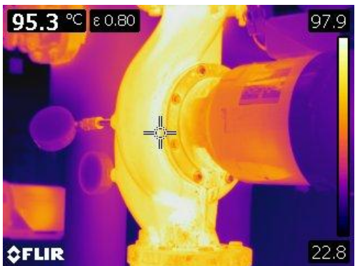
Figure 17 Thermographic image of motorized pump at 95.3° C or 203° F.
