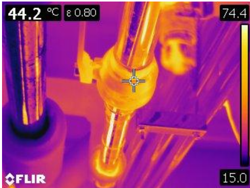
Figure 25 Thermographic image of bare copper piping at 44.2° C or 111° F.
