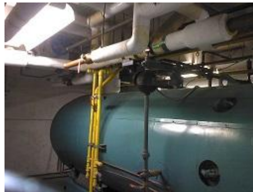
Figure 28 Conventional image of the same piping from boiler.
