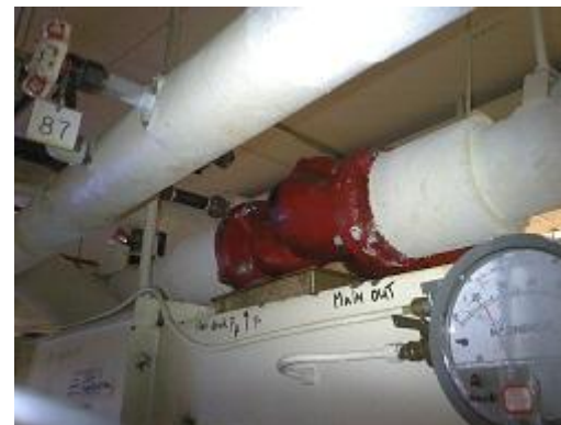
Figure 32 Conventional image of the same motorized heating pump.
