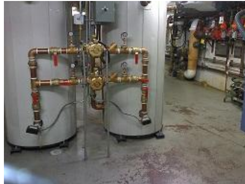
Figure 8 This is a conventional photo of the two heating pump and copper pipe at the hot water tank.
