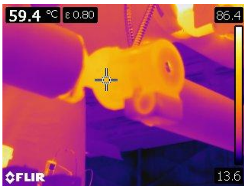
Figure 5 This Thermographic image of a re-circ pump adjacent to boilers.
