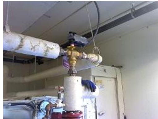
Figure 30 Thermographic image of the same bare motorized Tee.
