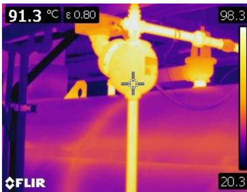
Figure 27 Thermographic image of pressure relief piping from the boiler at 91.3° C or 196° F.
