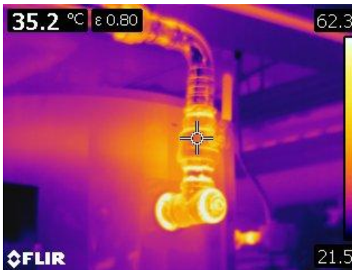
Figure 9 This is a thermographic image of copper pipe heating supply at 35.2° C or 95° F.
