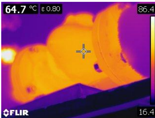
Figure 31 Thermographic image of bare motorized heating pump at 93.2° C or 199° F .
