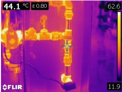
Figure 7 This is a thermographic image of copper pipe at the hot water tanks at 44.1° C or 111° F.
