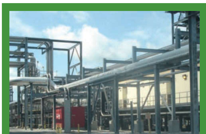
A utility pipe rack at Dow Chemical's St. Charles Operations in Hahnville, Louisiana.
