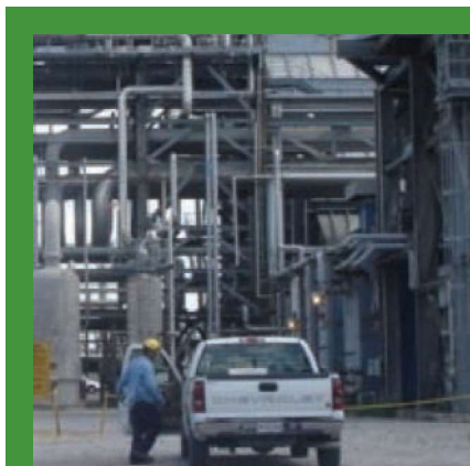
The east heat recovery unit at Dow's St. Charles Operations in Hahnville, Louisiana.
