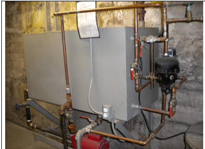
Figure 4. Uninsulated Condensate Tank in Corrections Building (14)
