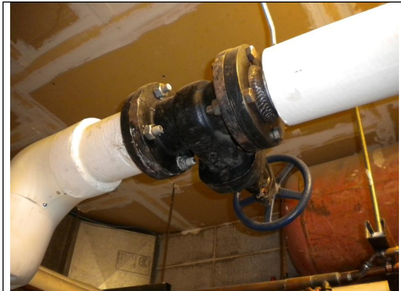
Figure 6. Uninsulated Steam Valve in Fish Wildlife and Parks Building (16)
