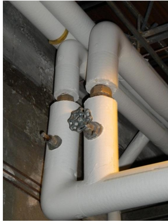
Figure 2. Uninsulated Unions and Valve Bonnets in HHW Lines
