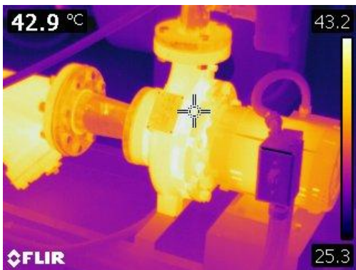
Figure 19 Thermographic image of a motorized pump and pipe at 42° C or 107° F.
