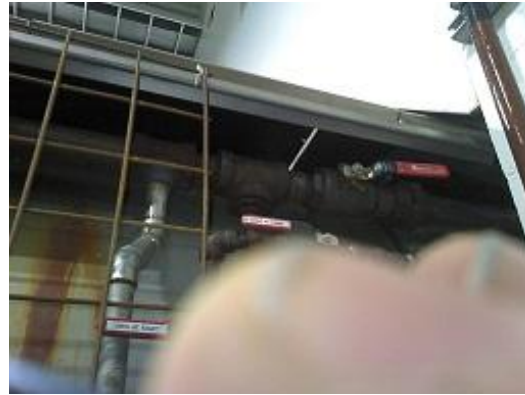
Figure 38 Conventional image of the same steam supply piping.
