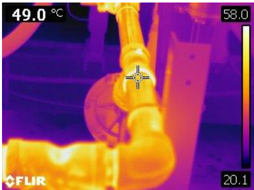
Figure 39 Thermographic image of a supply line at the bottom of the washers at 137° C or 278° F.
