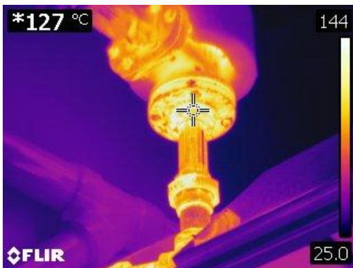
Figure 35 Thermographic image of steam supply to washers at 127° C or 260° F.
