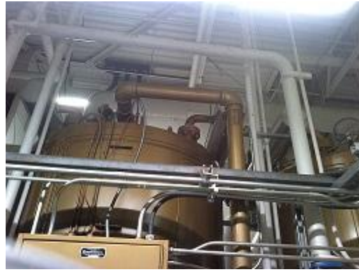
Figure 16 This is a conventional image of the same pipe at the top of the boiler.
