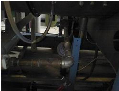
Figure 40 Conventional image of the supply line at the bottom of the washers.
