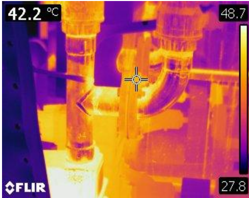
Figure 21 Thermographic image of bare piping and valves at 42° C or 107° F.
