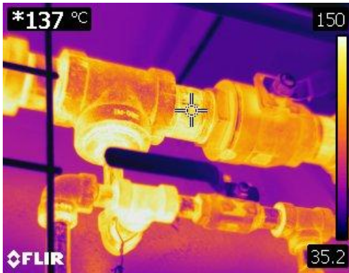
Figure 37 Thermographic image of a steam supply line to washers at 137° C or 278° F.
