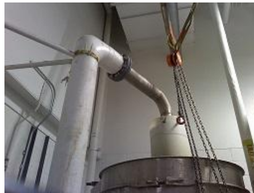
Figure 24 Conventional image of the same piping and flange.
