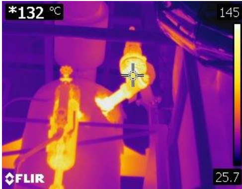
Figure 9 This thermographic image is of the sight glass and blow off/piping from this vessel at 132° C or 289° F.
