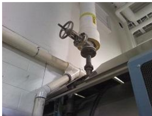
Figure 36 Conventional image of the same steam supply piping.
