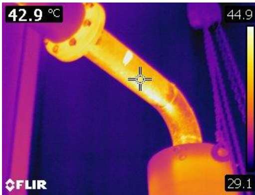
Figure 23 Thermographic image of bare piping and flange at 42° C or 107° F.
