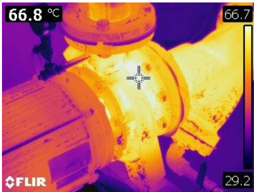
Figure 27 Thermographic image of bare pump and flange at 66° C or 150° F.
