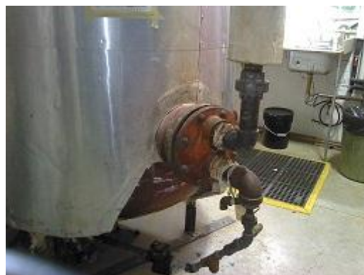
Figure 32 Conventional image of the same heat exchanger and piping.
