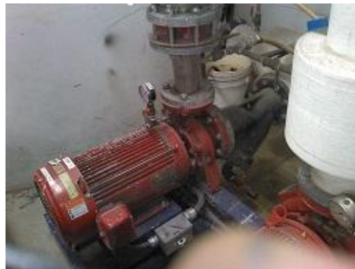
Figure 28 Conventional image of the same pump and flange.
