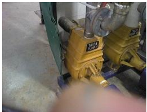
Figure 26 Conventional image of the same pump and flange.
