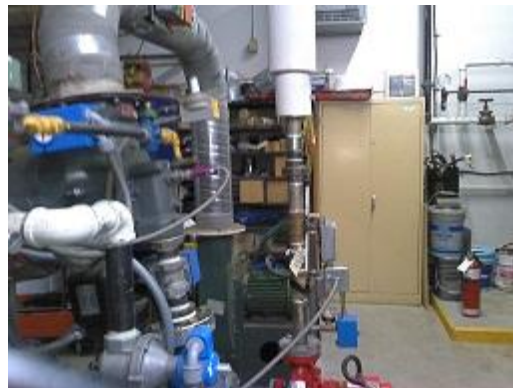
Figure 18 This conventional image is of the same pipe to the motorized pump.
