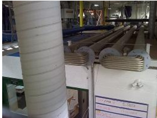
Figure 34 Conventional image of the same heat recovery piping.
