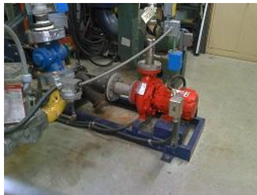
Figure 20 conventional image of the same pump and piping.
