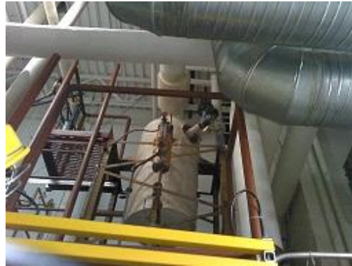
Figure 10 This is a conventional photo of the same sight glass and blow off/piping.
