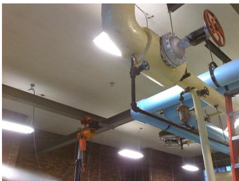
Figure 18 Conventional image of the same elbows and piping.
