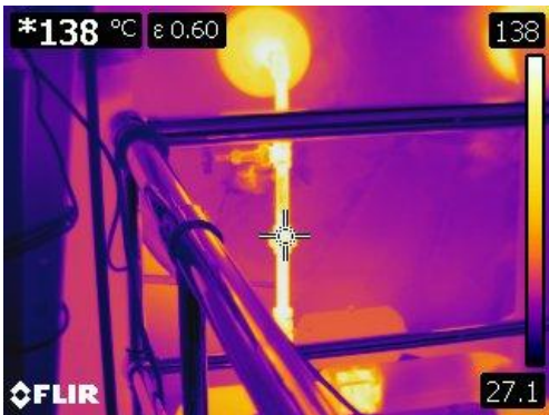
Figure 15 This thermographic image is of a bare pipe union at 138° C or 280° F
