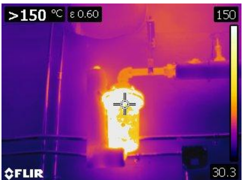
Figure 11 This is a thermographic image of a steam trap at a temperature greater than 150° C or 302° F.
