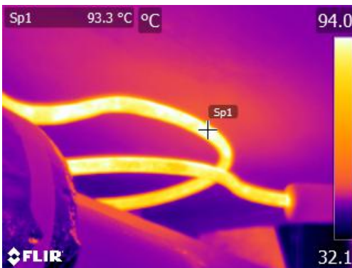
Figure 97 Thermographic image of uninsulated piping at 93.3° C or 200° F
