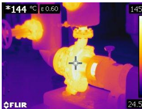
Figure 27 Thermographic image of pump at 144° C or 291° F.
