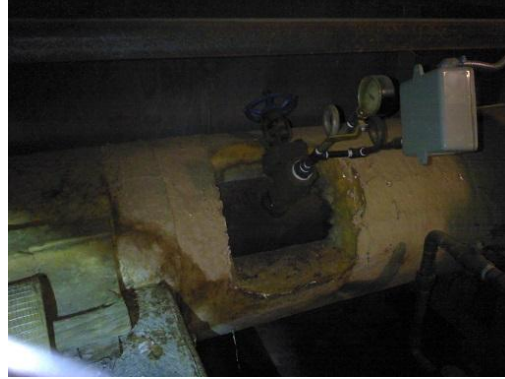
Figure 72 Conventional image of the same pipe and valve.
