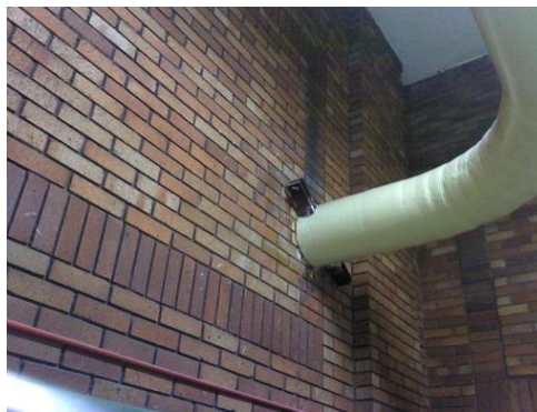
Figure 22 Conventional image of the same pipe support.
