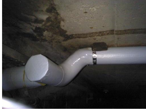
Figure 100 Conventional image of the same piping, note that the PVC jacketing on the material is melting.
