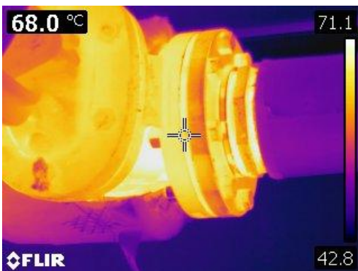
Figure 109 Thermographic image of an uninsulated valve at 68° C or 154° F
