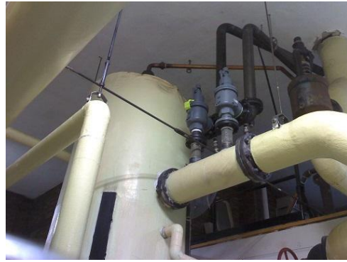
Figure 8 This is a conventional photo of the same piping and valve.
