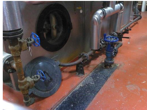
Figure 44 Conventional image of the same piping and flange.
