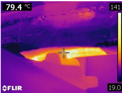
Figure 87 Thermographic image of an uninsulated roller support at 79.4° C or 175° F
