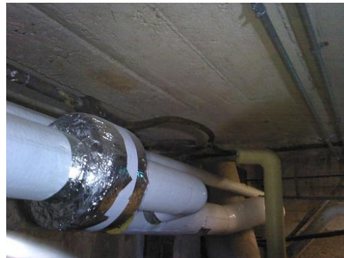
Figure 98 Conventional image of the same piping.
