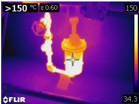
Figure 31 Thermographic image of a steam trap at a temperature greater than 150° C or >302° F.
