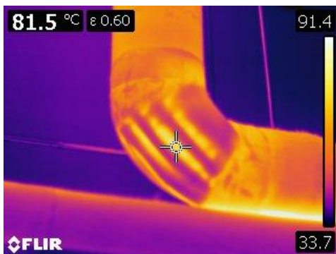
Figure 33 Thermographic image of an elbow with older fiberglass insulation and PVC covering at 81.5° C or 178° F.
