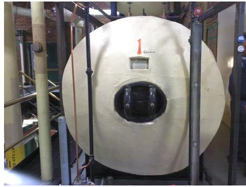
Figure 14 Conventional image of the same manway on tank.
