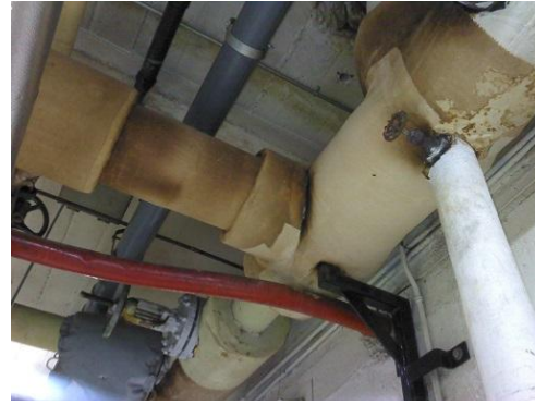
Figure 36 Conventional image of the same insulated piping. Note how the canvas is burned due to the heat.
