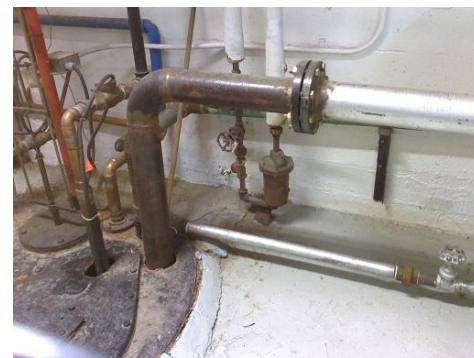
Figure 32 Conventional image of the same piping.
