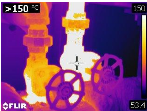
Figure 73 Thermographic image of uninsulated valves greater than 150° C or 302° F
