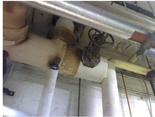
Figure 26 conventional image of the same valve bonnet. Note the burnt pipe covering.
