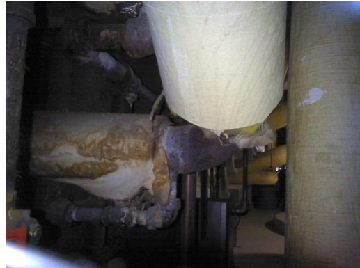
Figure 76 Conventional image of the same elbow.
