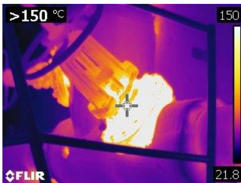
Figure 49 Thermographic image of bare valve bonnets and a pressure reducing valve at 119° C or 246° F
