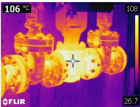
Figure 41 Thermographic image of bare valves at a temperature of 106° C or 223° F.
