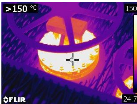
Figure 53 Thermographic image of a valve greater than 150° C or 302° F
