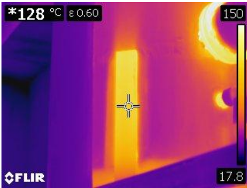
Figure 19 Thermographic image of the bare vessel support at 128° C or 262° F
