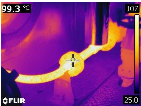
Figure 43 Thermographic image of bare pipe and flange at a temperature of 99.3° C or 211° F
