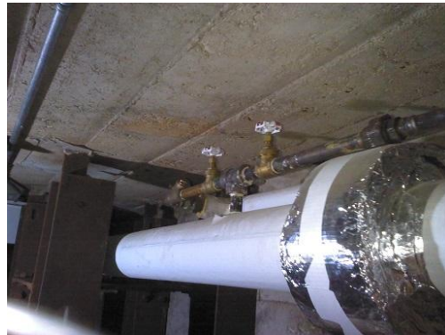
Figure 96 Conventional image of the same piping and valves.
