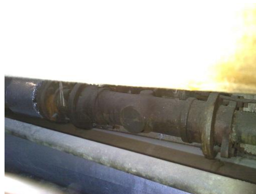
Figure 86 Conventional image of the same exchanger.
