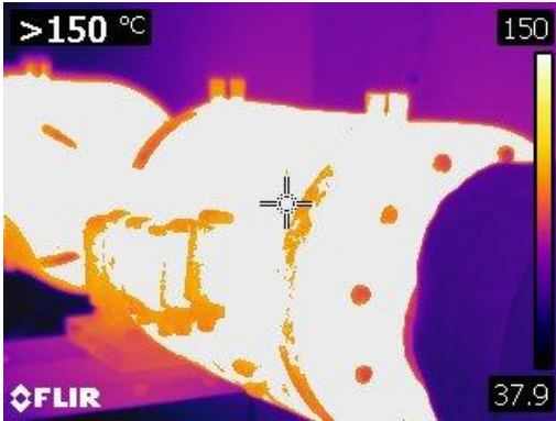
Figure 111 Thermographic image of an uninsulated expansion joint greater than 150° C or 302° F
