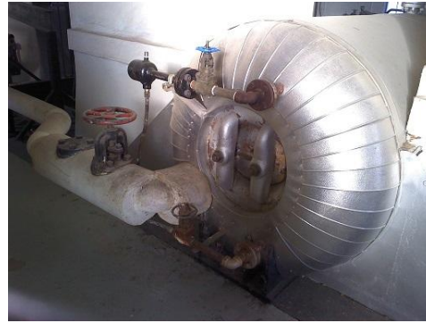
Figure 52 Conventional image of the same bare manway on the upper level of the furnaces.
