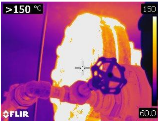
Figure 61 Thermographic image of bare flange greater than 150° C or 302° F
