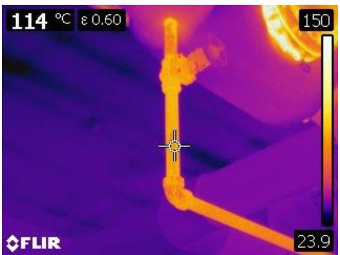
Figure 17 Thermographic image of unfinished elbows and piping at 114° C or 237° F
