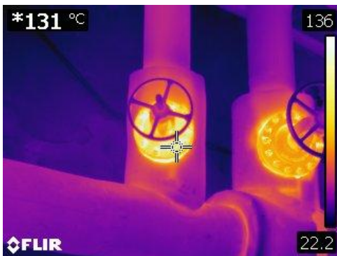
Figure 47 Thermographic image of bare valve bonnets at 131° C or 267° F.
