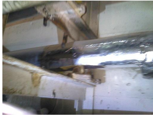
Figure 88 Conventional image of the roller support.
