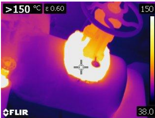
Figure 25 Thermographic image of a valve bonnet at a temperature greater than 150° C or >302° F.
