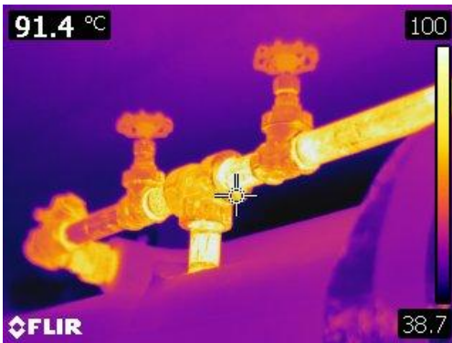
Figure 95 Thermographic image of bare piping and valves at 91.4° C or 197° F
