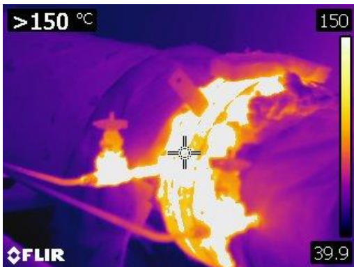
Figure 57 Thermographic image of bare flange and small valve greater than 150° C or 302° F
