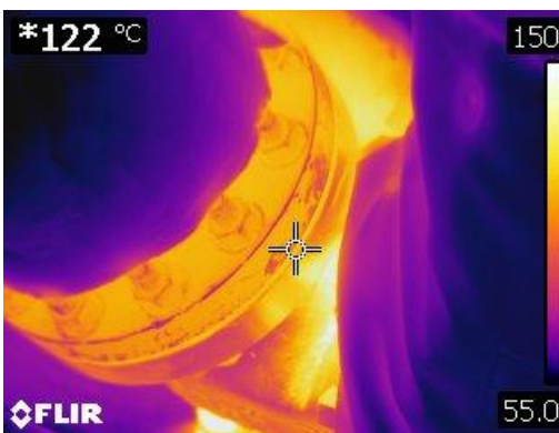
Figure 65 Thermographic image of bare valve at 122° C or 252° F.
