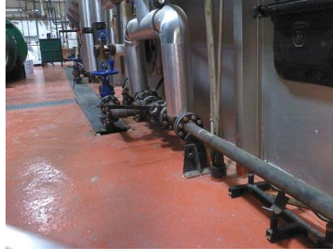
Figure 46 Conventional image of the same piping.
