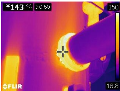
Figure 9 This is a thermographic image of bare flange in the powerhouse at 143° C or 290° F.
