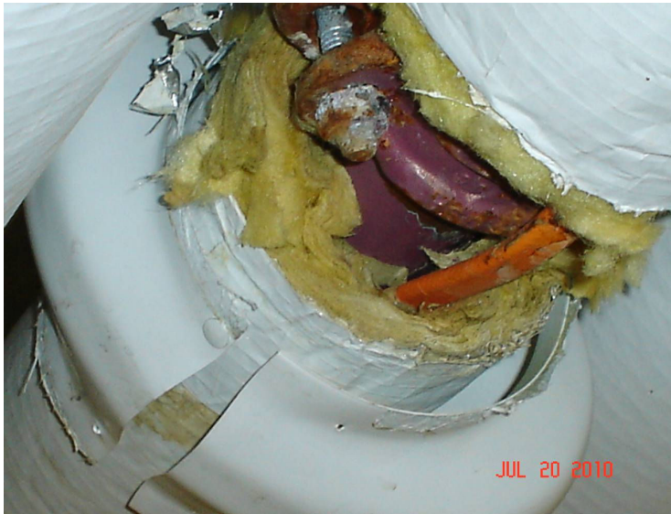
Corrosion and condensation in new LEED platinum condominiums in Vancouver.
