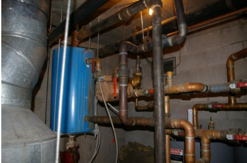
Photo 2 Detail showing un-insulated hydronic distribution system and heat exchanger for domestic hot water system
