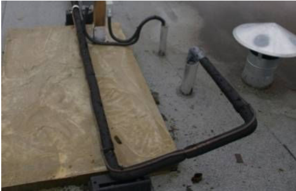
Photo 6 Detail showing rubber insulation on a hot gas refrigerant line. The insulation should be jacketed to protect it from sun and birds.
