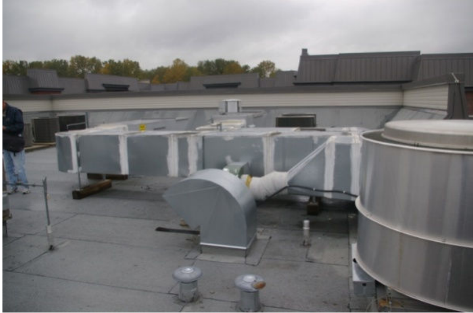
Photo 7 Detail showing a section of an un-insulated supply air duct on a roof mounted make-up air unit.
