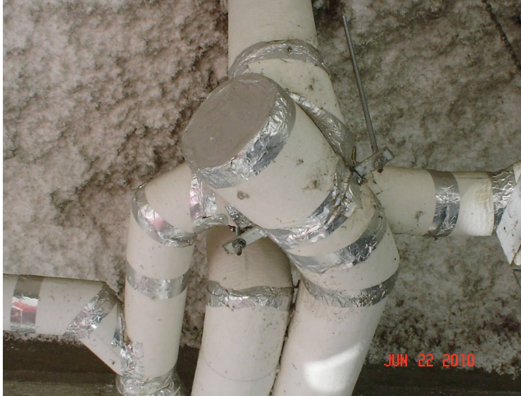
Poorly finished pipe covering in an outdoor parkade. No weather proof jacketing or elbows.
