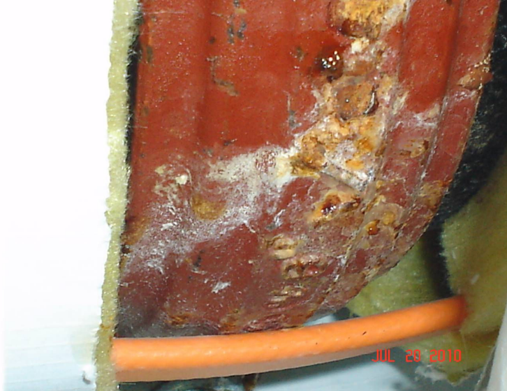
Corrosion and condensation in new Vancouver condominiums.
