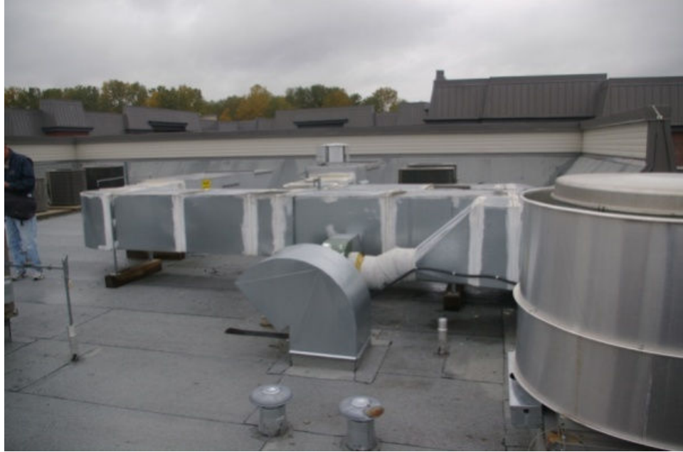
Photo 7 Detail showing a section of an un-insulated supply air duct on a roof mounted make-up air unit.
