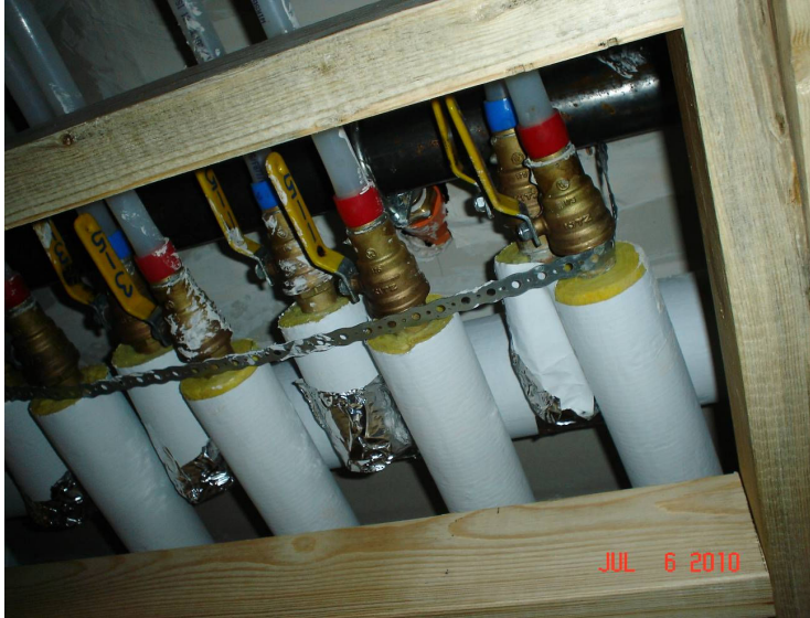
Incomplete domestic water pipe insulation in unfinished condominiums in Vancouver.
