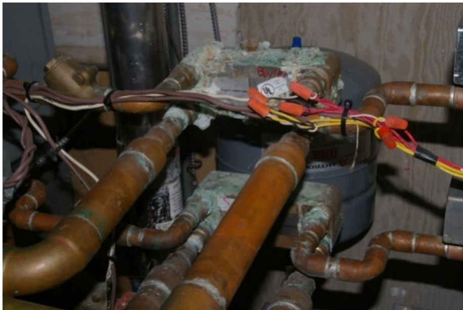
Photo 5 Detail showing heat exchangers used with domestic water system approximately 12 years old. Note the build up of deposits on the heat exchangers.
