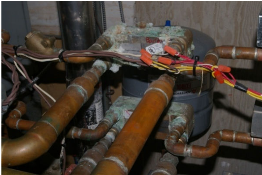
Photo 5 Detail showing heat exchangers used with domestic water system approximately 12 years old. Note the build up of deposits on the heat exchangers.
