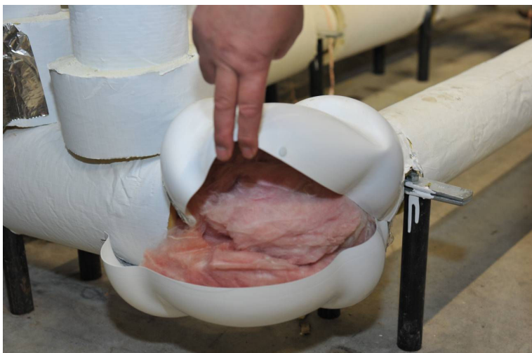
An example of an improper system with no vapour barrier and use of pink insulation instead of a matched density flexible insulation equivalent to the adjacent pipe covering.
