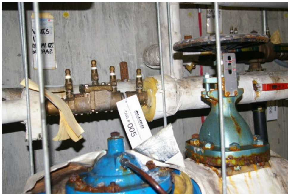
Photo 3 Detail showing backflow preventer on domestic water supply line. Note the water dripping from the device.
