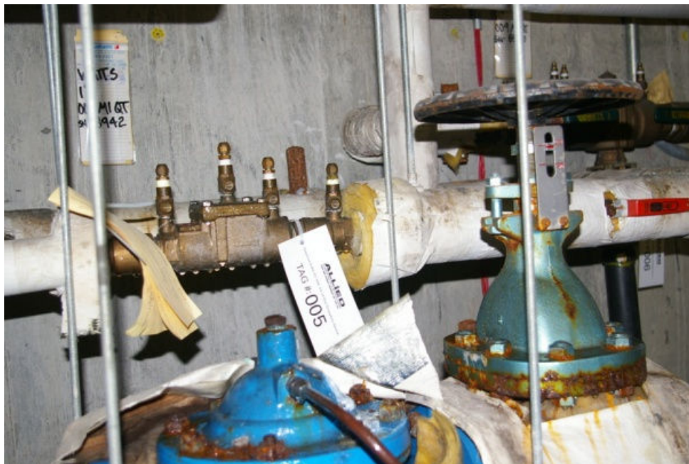
Photo 3 Detail showing backflow preventer on domestic water supply line. Note the water dripping from the device.
