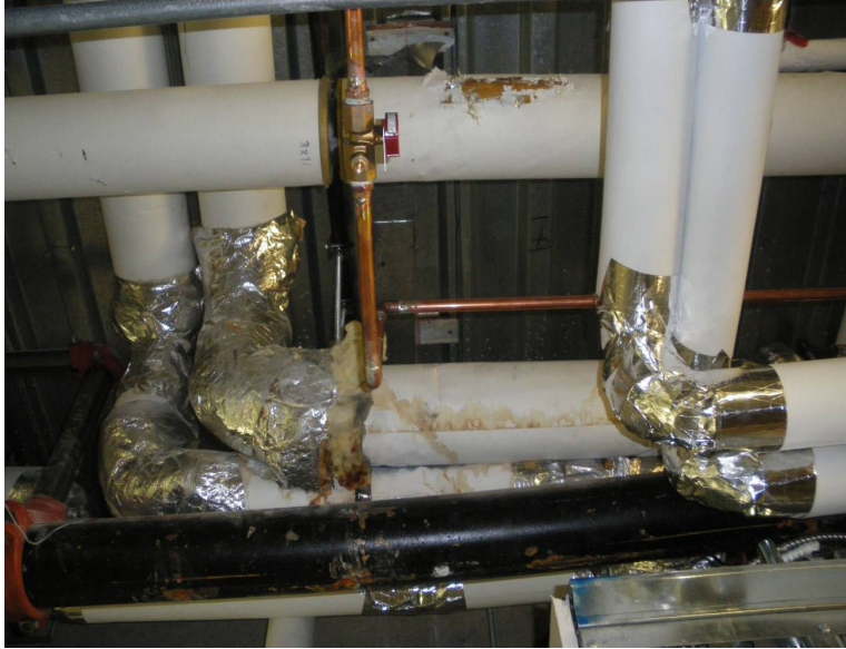
Further evidence of sweating and corrosion at a medical facility. Note that even though the insulation appears to be sealed along the longitudinal seam, the poor quality insulation vapour barrier is not performing as it is supposed to.
