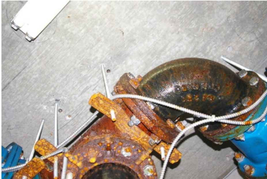
Photo 4 Detail showing corrosion damage to pipe fittings as the result of condensation.
